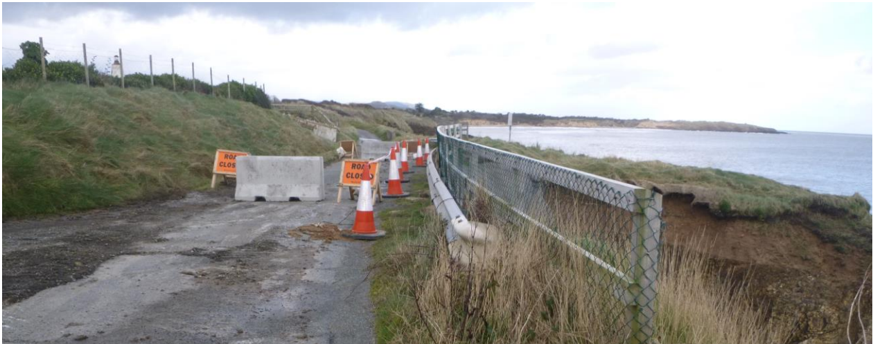
Closed sea road in N County Wexford as erosion threatens. Picture by Paul Dubsky.
