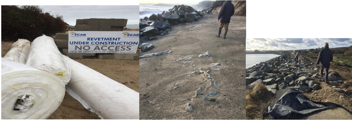
Figure 28. Geotextile are all over the places – Photos by Karin and Paul Dubsy
